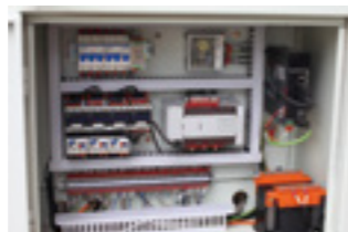
Precise control of electrical components
