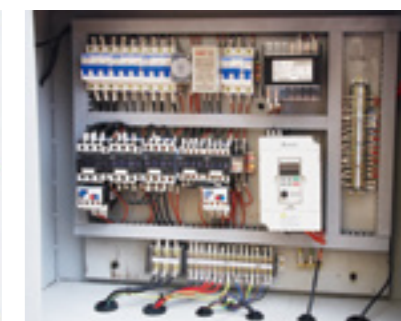
Electrical control box
